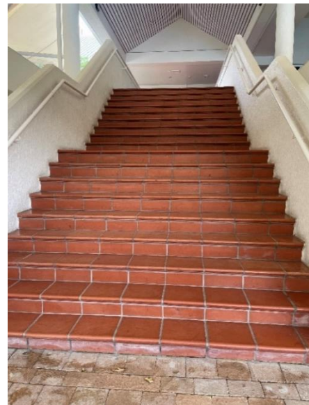
Photo of staircase without hi-vis step markings
