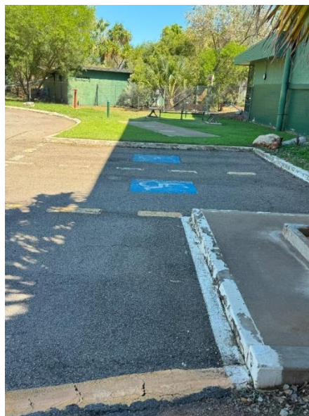
Photo showing no tactile markings to indicate where roadway starts and uneven ground
