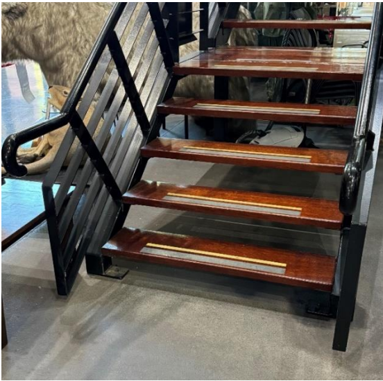
Photo of internal stairs with no tactile markers
