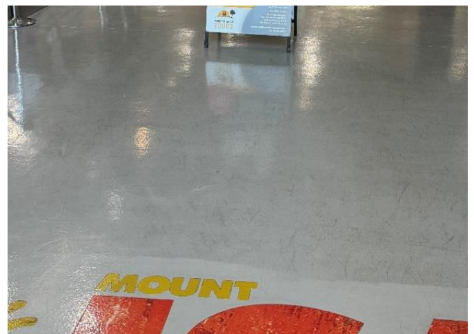
Photo of smooth surface on the floor – tripping hazard if wet
