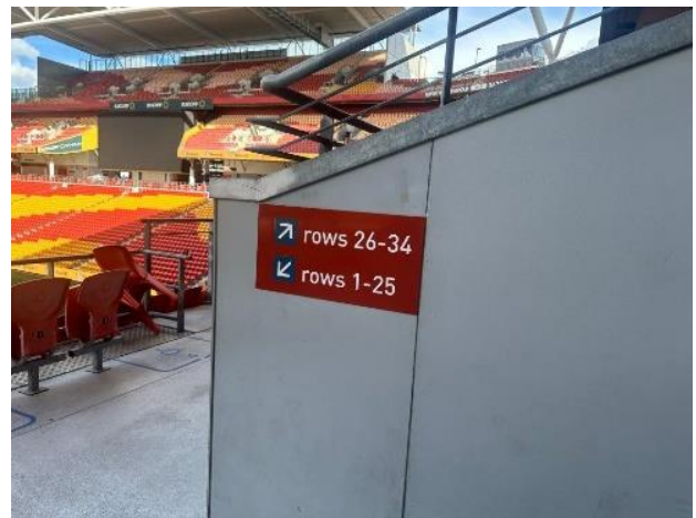
No Braille or tactile directional signage, although what is provided is shows good colour contrast.
