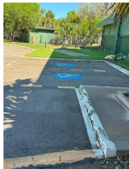
No tactile markings to indicate where roadway starts and uneven ground
