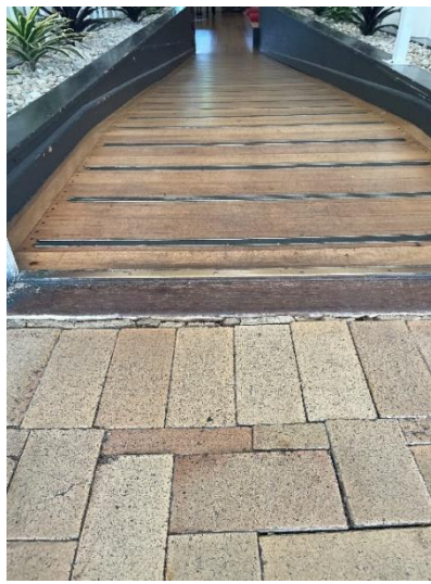
Ramp without even step / no hi-vis marking
