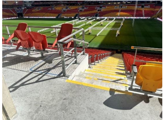
Stairs to seats would benefit from a repaint of the colour contrast. No TGSIs.
