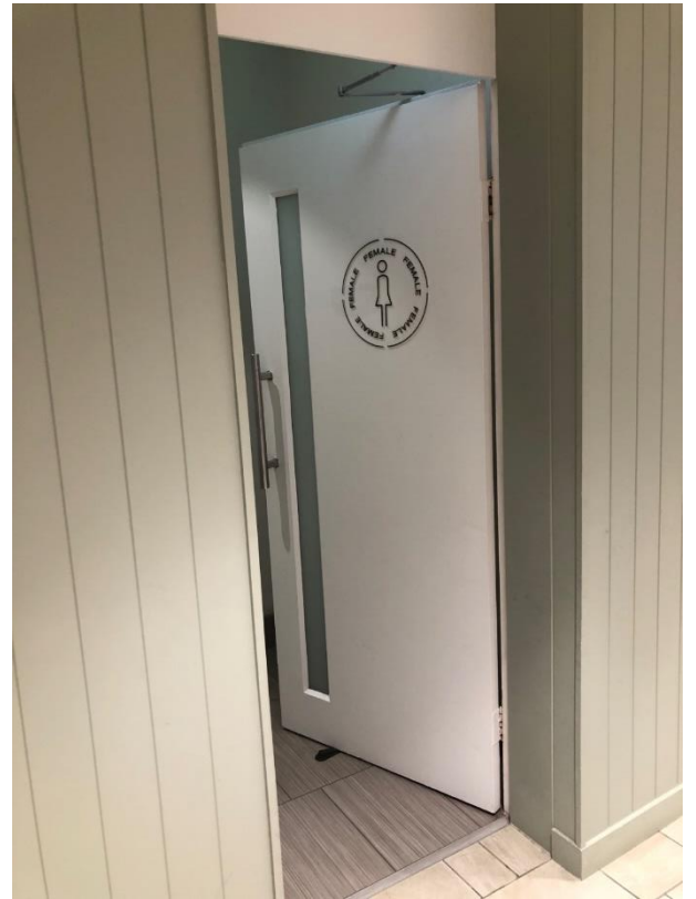
Signage is on the door, and the door is open. No braille, and the tactile symbol is unrecognisable
