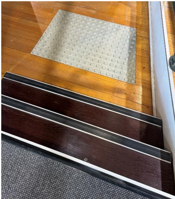
Tactile markers indicating stairs, as well as colour contrast stair tread strips
