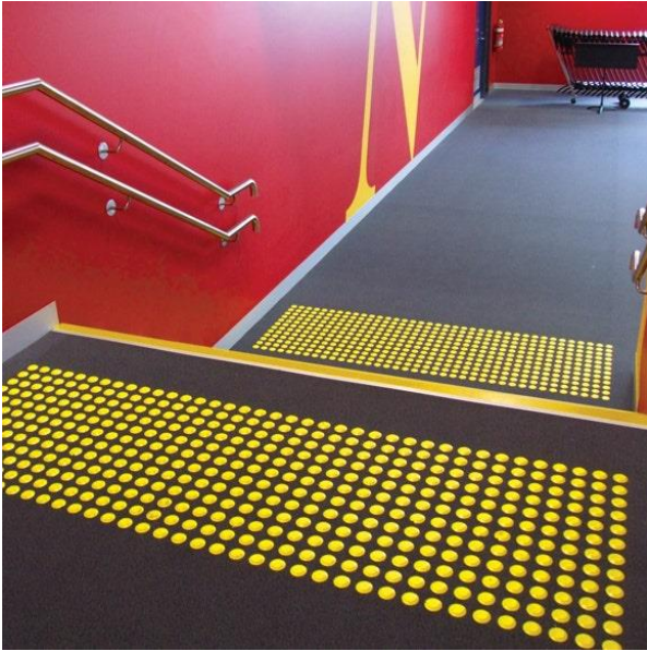
Stairs with high-contrast nosing on tread and riser, and TGSIs at the top and bottom. https://www.bronsonsafety.com.au/
